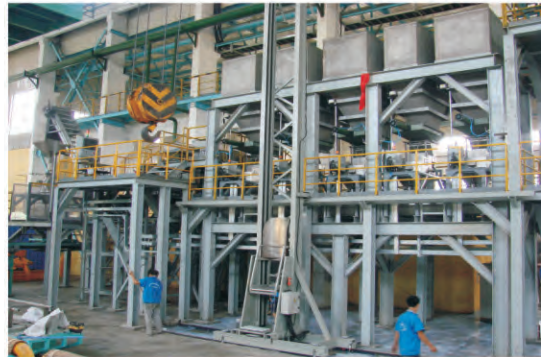
automatically weighing and mixing system
